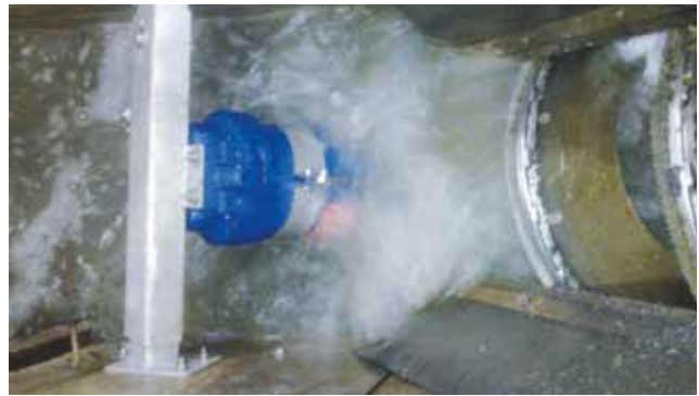
External screenings washing system (ERGA). A preceding washing system washes out the organic matter.
