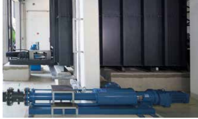
Sludge bunker and pump.
