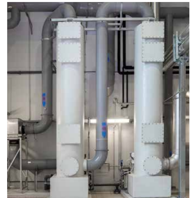
Two stage scrubber for odor control.
