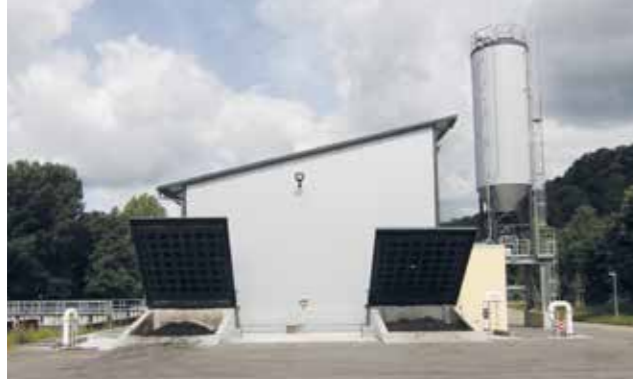
Sludge bunker and dry material silo.
