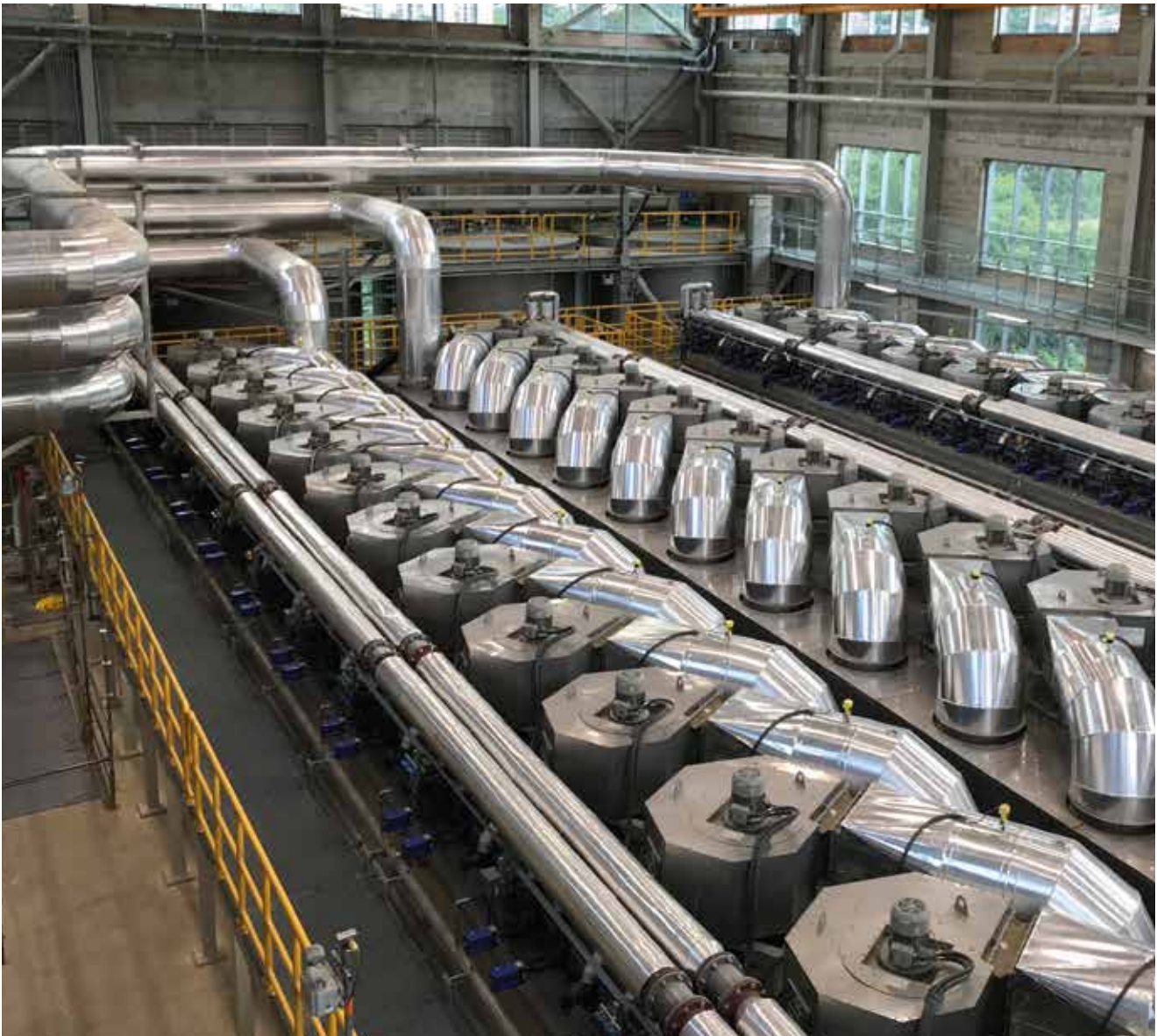
Multi-line design of the HUBER Belt Dryer BT for large projects.
